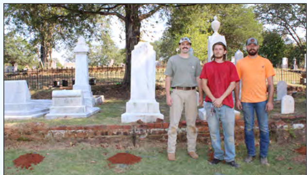
The Ensley Iron, LLC crew during installation of the new wrought iron fence. (L-R) Adam Ducote, Alex Little, Mathew McCurry.
