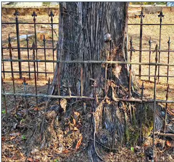
Two large trees bordering the plot had grown into sections of the old fence. Ensley Iron expanded the footprint of the plot with the new fence allowing the sections "eaten by the trees" to be left intact as an artifact from the past.
